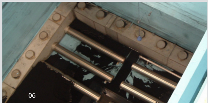
04 Off-set effluent collection/backwash water header 05 Center eductor 06 Sub-fluidized exhausted GAC media automatically educted from the basin
